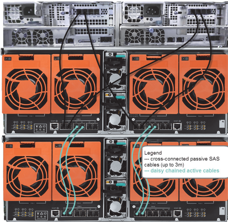
Unity 3300 connected to U2G460 expansions
